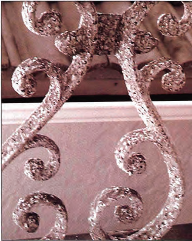
This scroll casting is not marine grade. It shows severe white corrosion after only 18 months in its ocean environment in Sarasota, FL. No coating remains.
