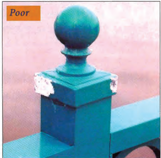
This 2" ball cap is not marine grade. It shows chalk corrosion and flaking (starting at corners) after four years on the Indian River in Vero Beach, FL.
