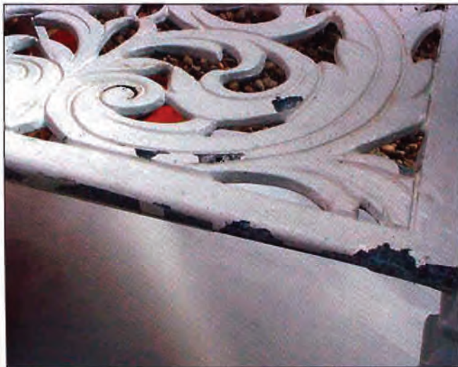
This 12-year-old aluminum furniture in Dallas, TX, is also not marine grade. Even though it is not in a harsh marine environment, its powder coat is peeling and corrosion appears.
